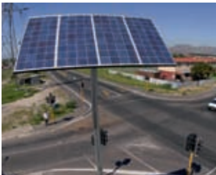
SOLAR-POWERED TRAFFIC LIGHTS, LOTUS RIVER
