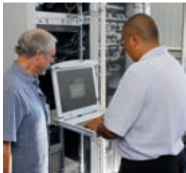
IT SYSTEM - PAUL SAUER BUILDING
